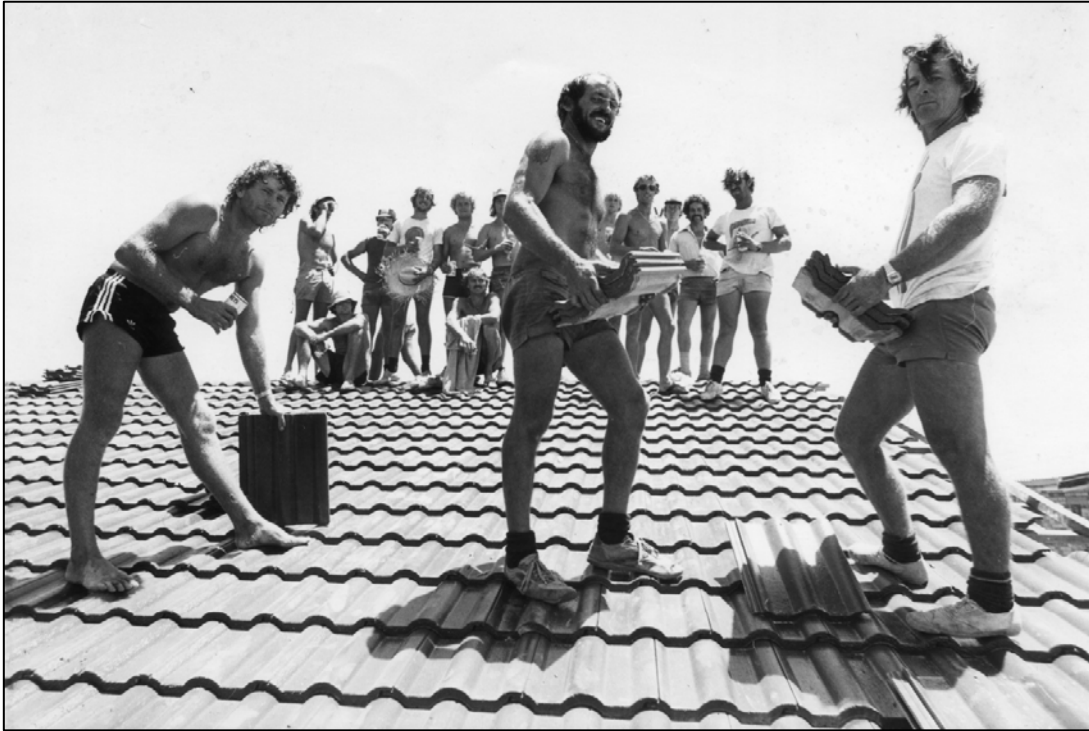
First tiling of the roof the current Sawtell Surf Life Saving Clubhouse in 1982
